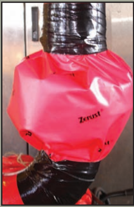
Offshore Platform - Fire Water Line
