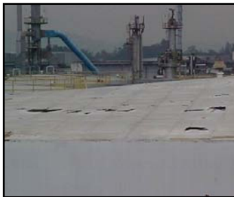
HOLES IN THE ROOF OF AN AST
